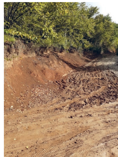
Slika 7. Erozija kosina iskopa Figure 7. Erosion of the excavation slope
